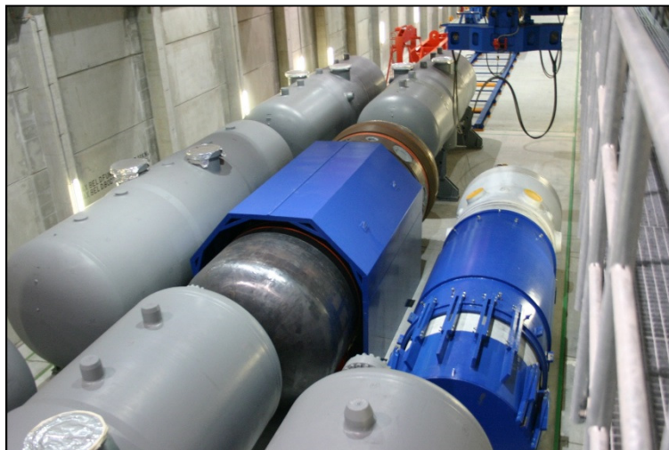
Decay storage of unsegmented steam generators and RPVs at Interim Storage Facility Greifswald (ZLN) Source: EWN GmbH
