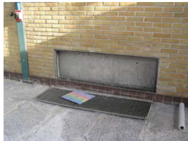
Figure 21. The heating air outlet from the reactor hall. The ventilation grills have been removed for measurements behind the grill and in the ducts.
