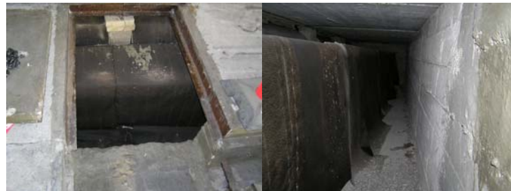
Figure 22. One of the channels with the ventilation ducts. To the left, the access to the channel is shown. To the right, the channel is seen. The channel has a height of 90 cm.
