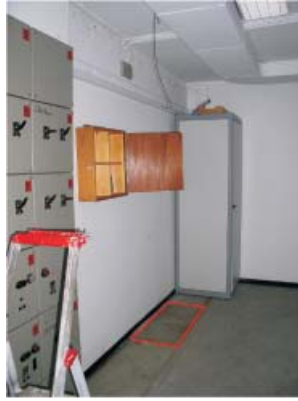
Figure 5. The landing of the stairway in the western basement. The area where the cupboard with the radioactive sources was situated is marked in red.
