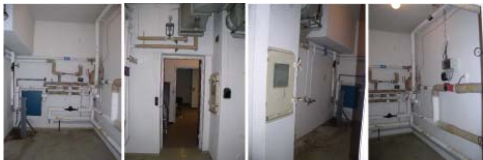
Figure 3. Room for heat control in the western basement.
