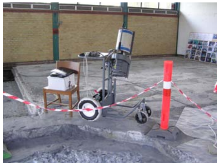
Figure 28. The measurement at the north-eastern part of the area where the biological shield was situated.
