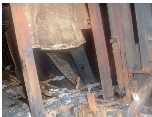
Figure 2. Portion of galvanised sidewall that was cut through by fire crew to facilitate access to the production line area
