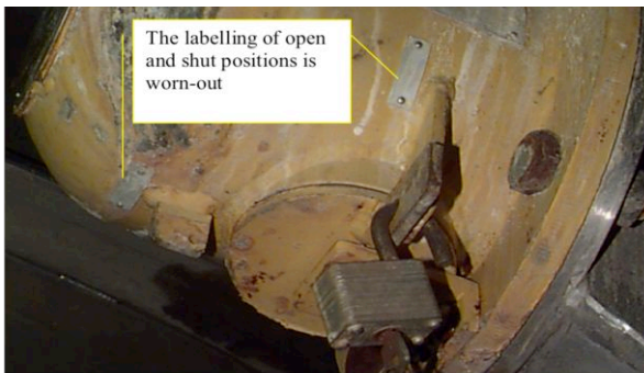
Figure 5: The labelling of open and shut position is worn-out.
