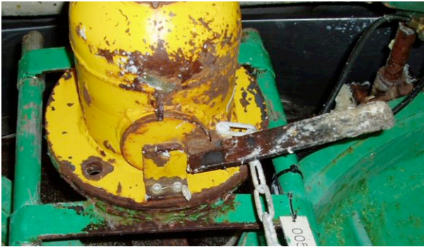
Figure 4: Rusty radionuclide gauge with extended handle
